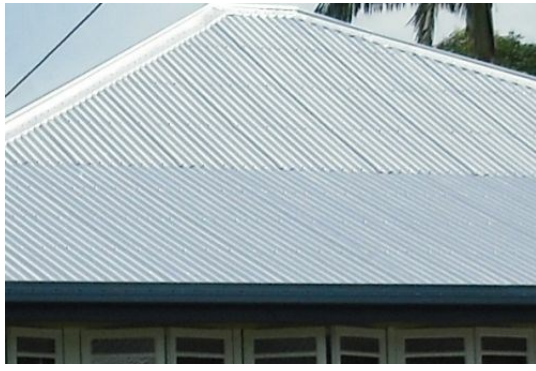
Figure SC6.2.3.22 Corrugated galvanized iron is typical for roofing in Townsville Character buildings
